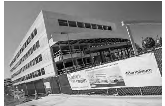
The entranceway takes shape at the new Ambulatory Care Center under construction at Skokie Hospital.
